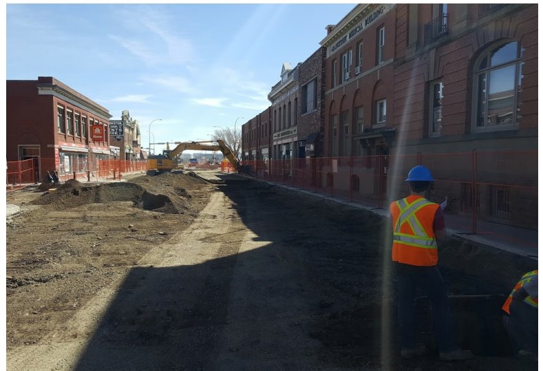
Above: Beginning with the removal of asphalt, it will take 4-5 weeks to replace the sanitary main in Stage 2 before the sidewalk replacement is complete in Stage 1 and the concrete crew advances into Stage 2.
